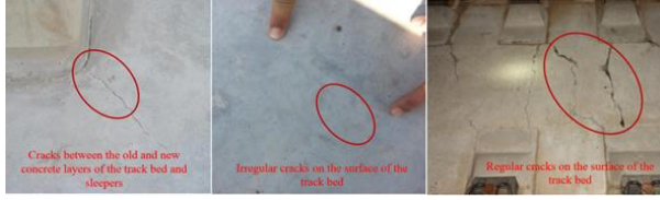
Fig. 1 Cracking in track bed concrete
