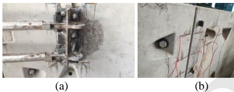
Fig. 12 Comparison of concrete damage on the internal side of the segmental joint: (a) Specimen 1; (b) Specimen 2
